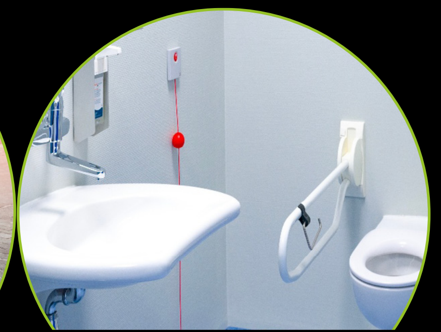
DISABLED TOILET ALARM SYSTEMS (DTA)
