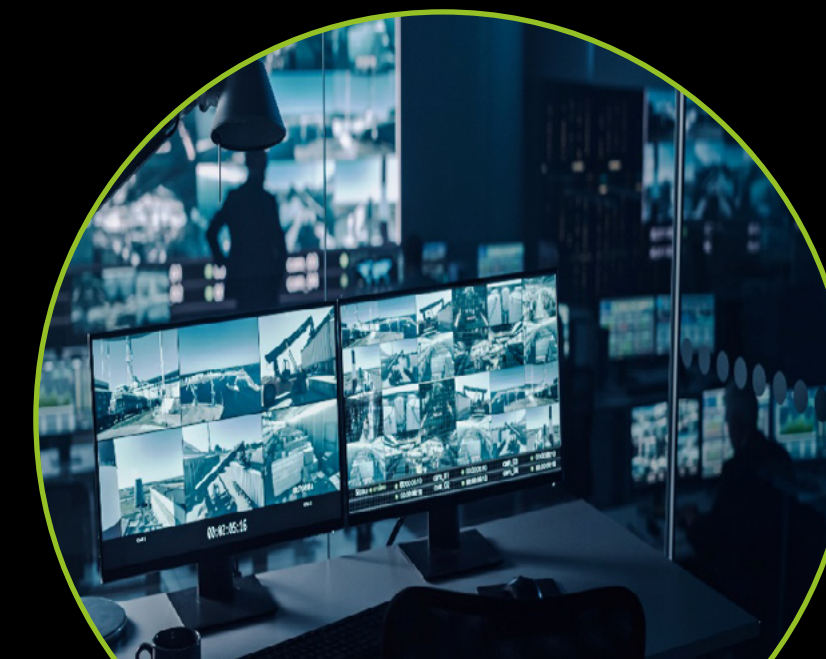
INTEGRATED SECURITY MANAGEMENT SYSTEM (ISMS)
